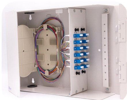
Outside Panel Wall box
